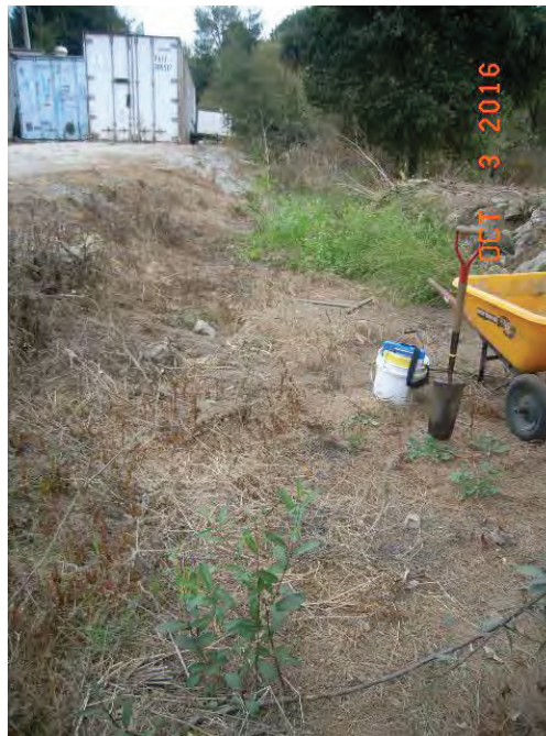
Figure 6. Condition of drainage swale, October 2016
